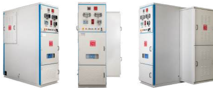
22KV VCB Panel - Overall View
