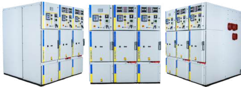
11KV VCB Panel - Overall View
